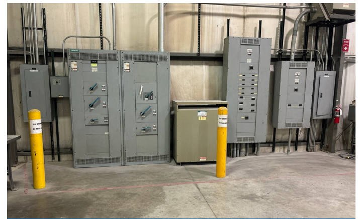
One of 2 Electrical Banks
